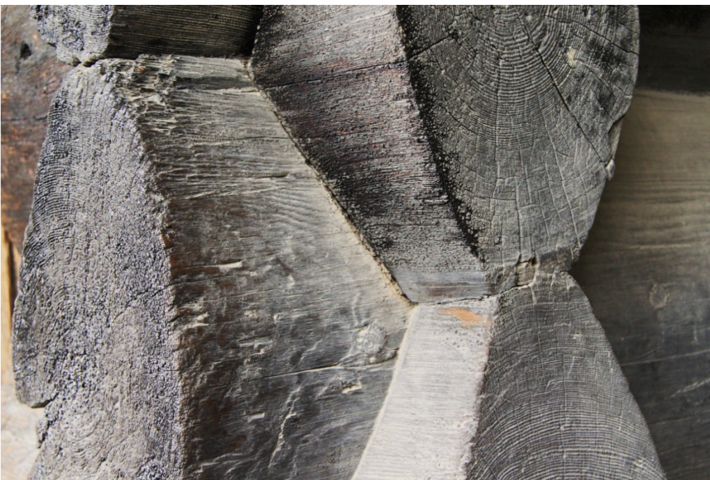
Fig. 2 – Detail of the medieval farm building located in the same Norsk Folkemuseum. The interlocking of horizontal beams can be seen.
